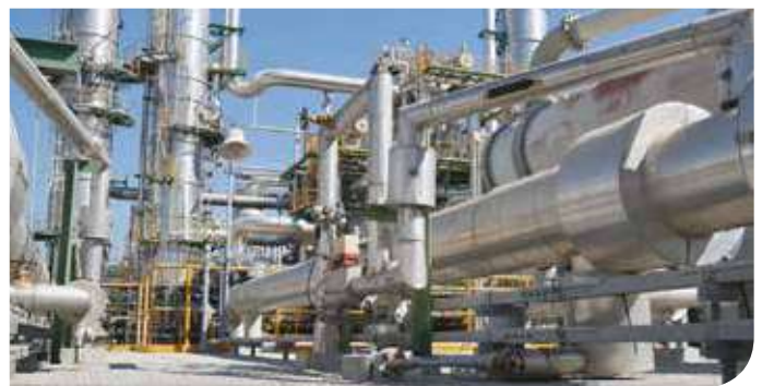
Oil Refinery Plant
