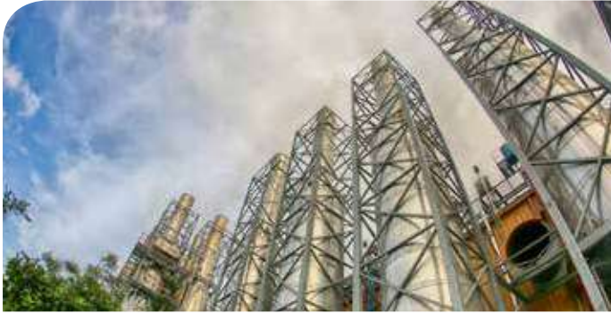
Power Generation Plant
