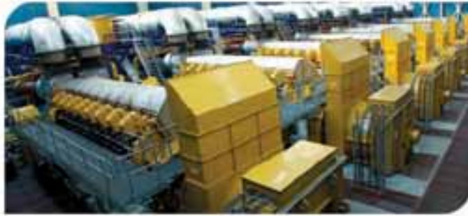
Power Generation Plant
