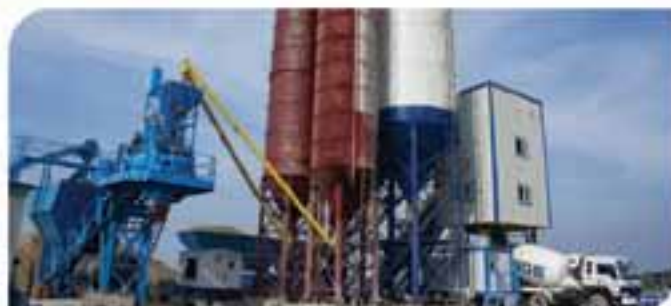
Ready Mix Processing Plant
