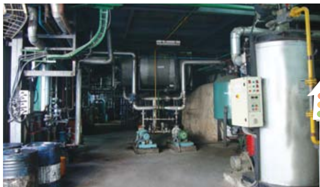
lube oil recycling plant
